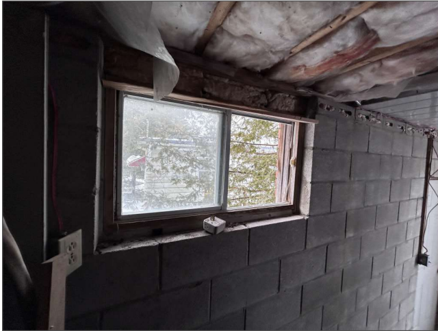
Double glazed IGU (basement)
