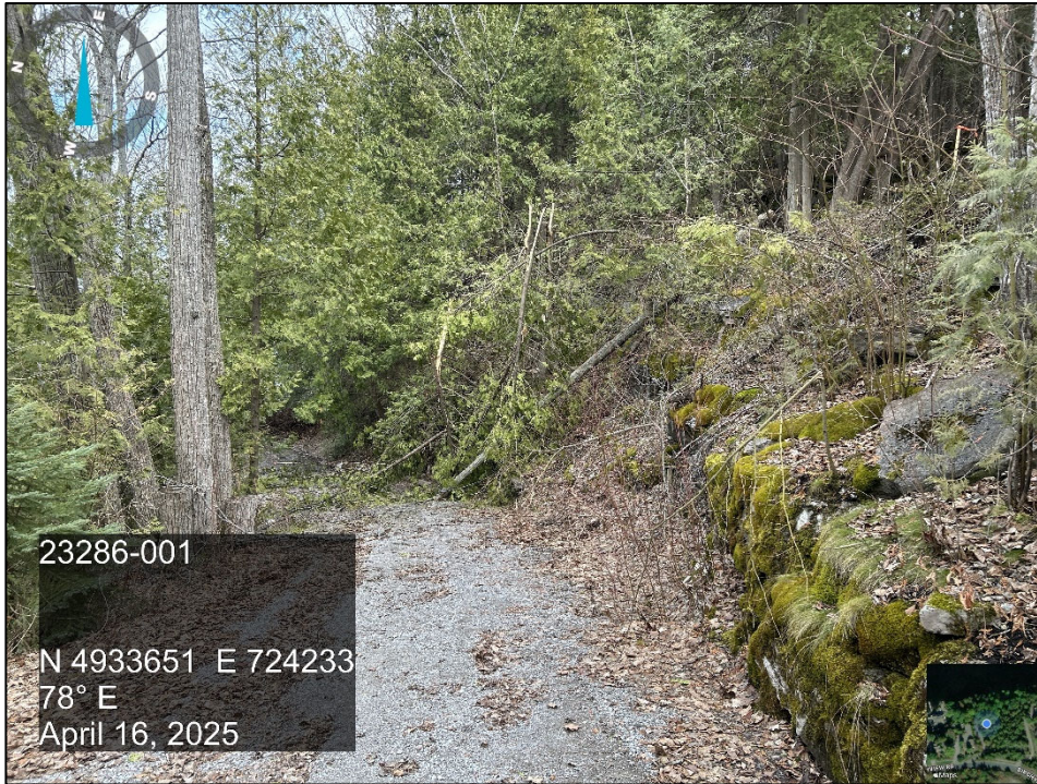
Photo 11 View of middle slope face near Cross Section B-B, looking east, showing the driveway, exposed bedrock, and mixed mature trees.
