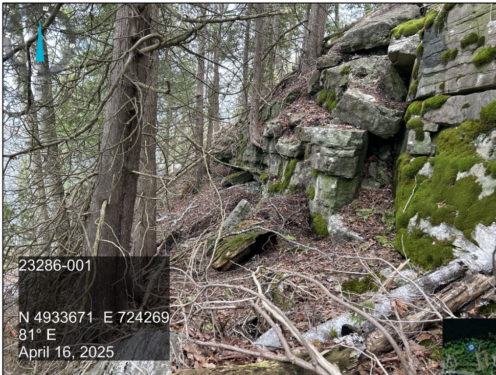
Photo 18 View of middle slope face near Cross Section C-C, looking east, showing exposed bedrock and mixed mature trees. Loose surficial rock is evident on top of the bedrock.
