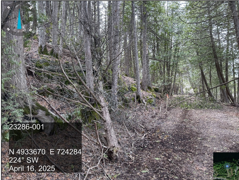
Photo 23 View of upper slope face near Cross Section D-D, looking southwest, showing loose surficial boulders and mixed mature trees.
