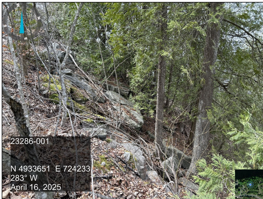
Photo 2 View of middle slope face near Cross Section A-A, looking west, showing loose surficial boulders and mixed mature trees.
