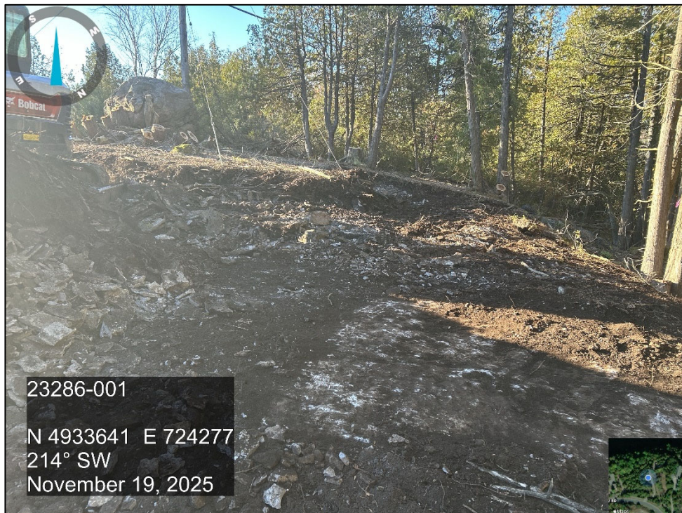
Photo 30 Test pits excavated along the top of the upper slope face near Cross Section C-C. Showing limestone bedrock with few joints beneath the loose surficial rock.
