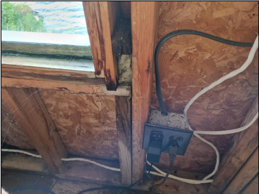
Photo 5 – Leaking Around Window Framing
