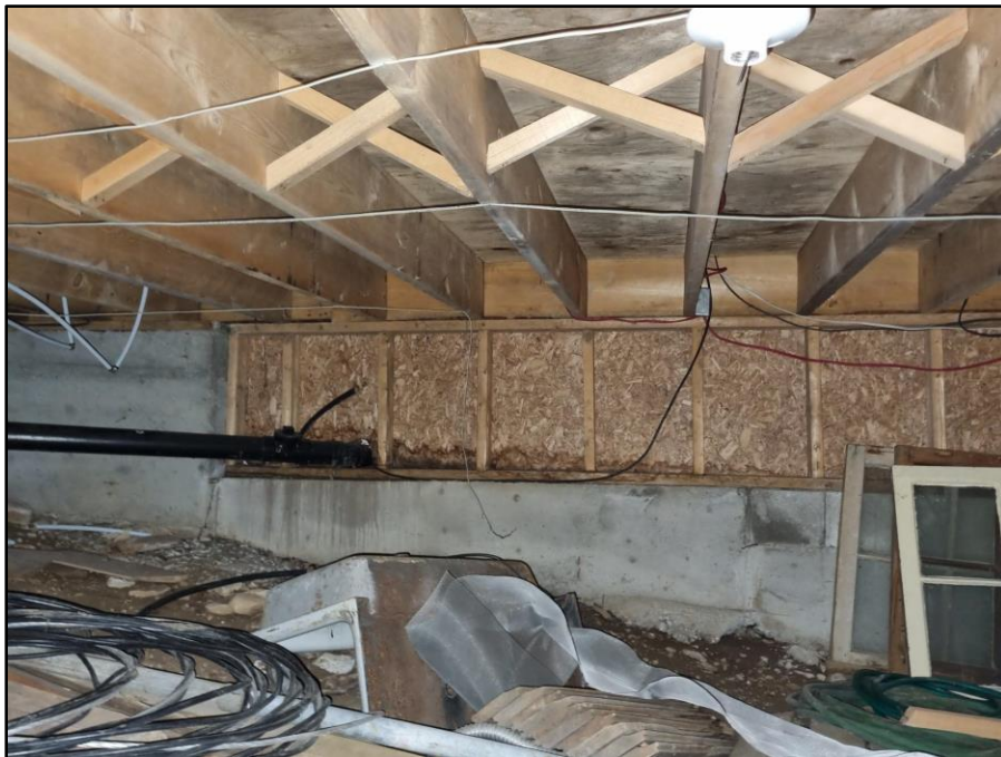
Photo 3 – Water Damage in Crawlspace
