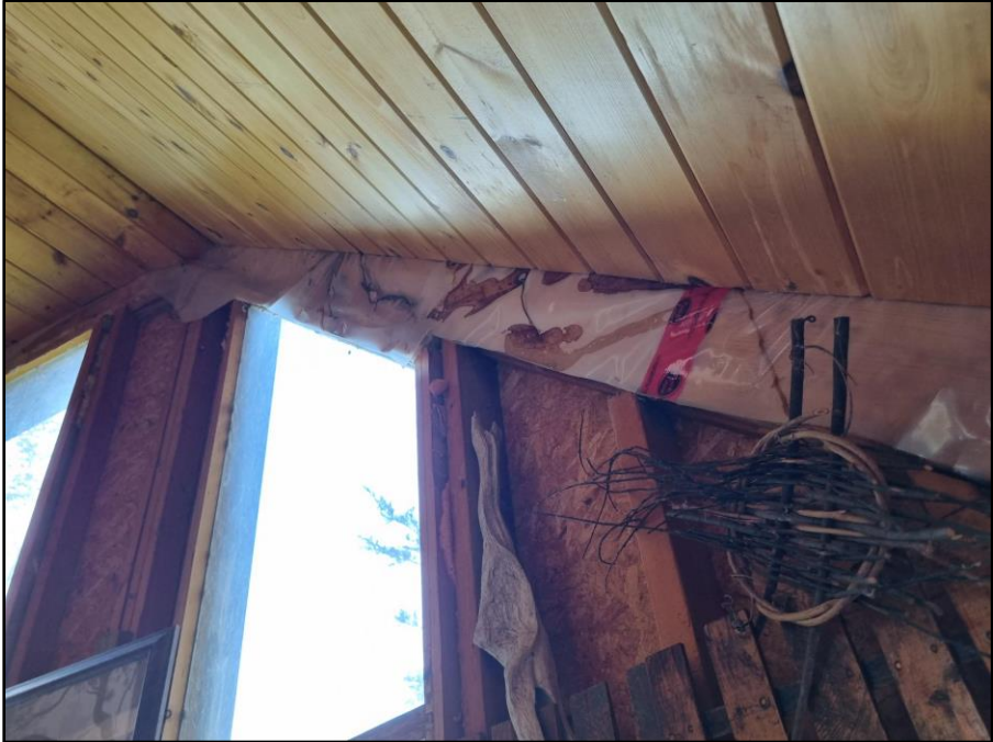
Photo 4 – Leaking from Ceiling into Wall Framing
