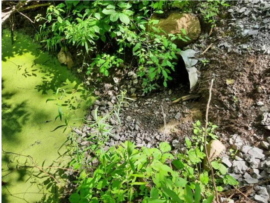
Photo 7 Perched steel culvert inlet crossing the western laneway, August 2022.
